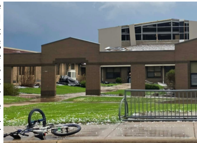
Damage to stage wall at Elementary School
